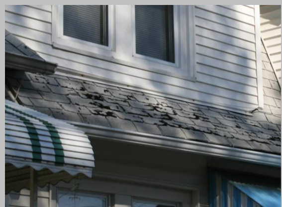
Deteriorated shingles such as these no longer serve their purpose of protecting the underlying roof structure.
