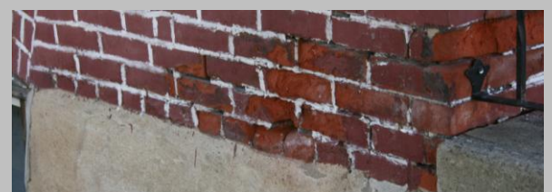
Moisture is the most significant cause of decay in masonry. Seen here are examples of mortar loss, efflorescence (salt leaching), and spalling (exploded face), all caused by excessive moisture.
