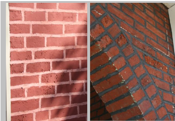
Never sandblast or use high-pressure power washing to clean masonry. Doing so can compromise the building structure by scarring masonry surfaces beyond repair, which will allow excessive moisture into the masonry. Note the pitting of these brick units that have witnessed abrasive cleaning.
